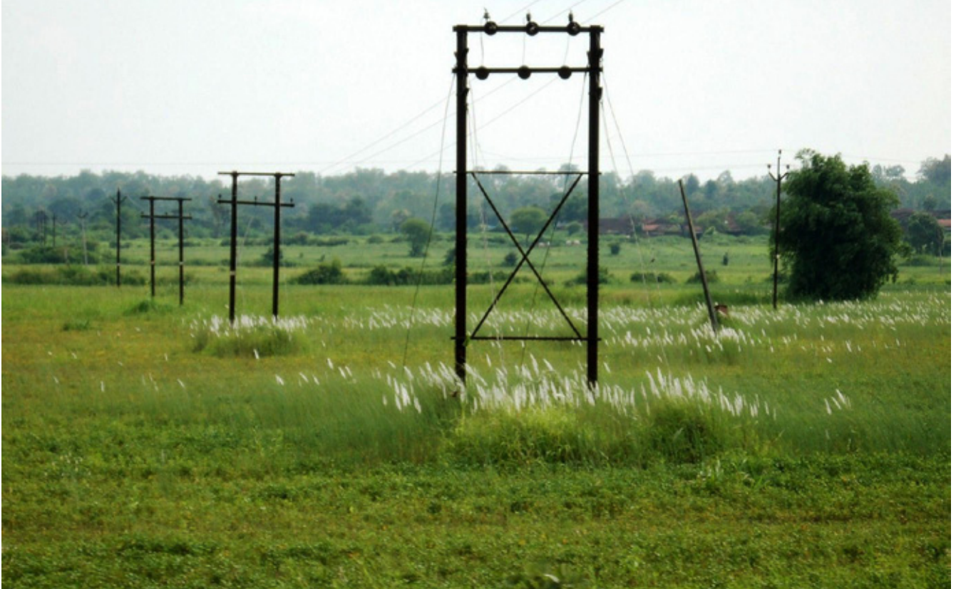
Electricity tower in Nagpur, India. Photo credit: Harshad Sharma, Flickr, Creative Commons.
