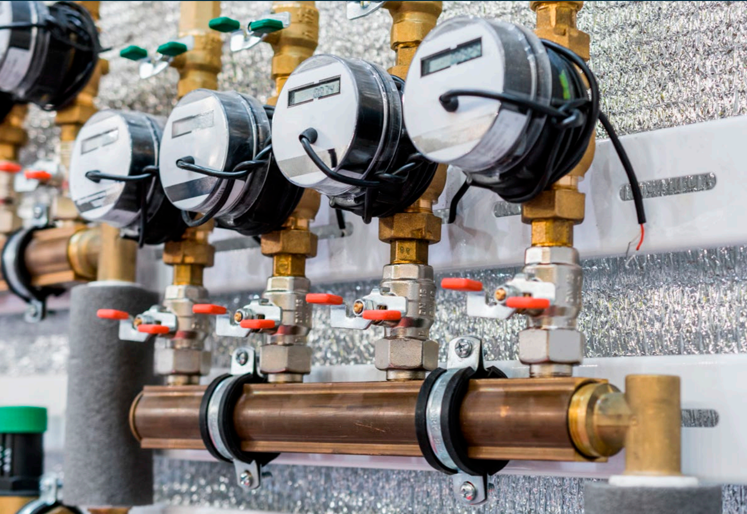
Several water meters. Measurement of water flow, Nordroden/Shutterstock.com.
