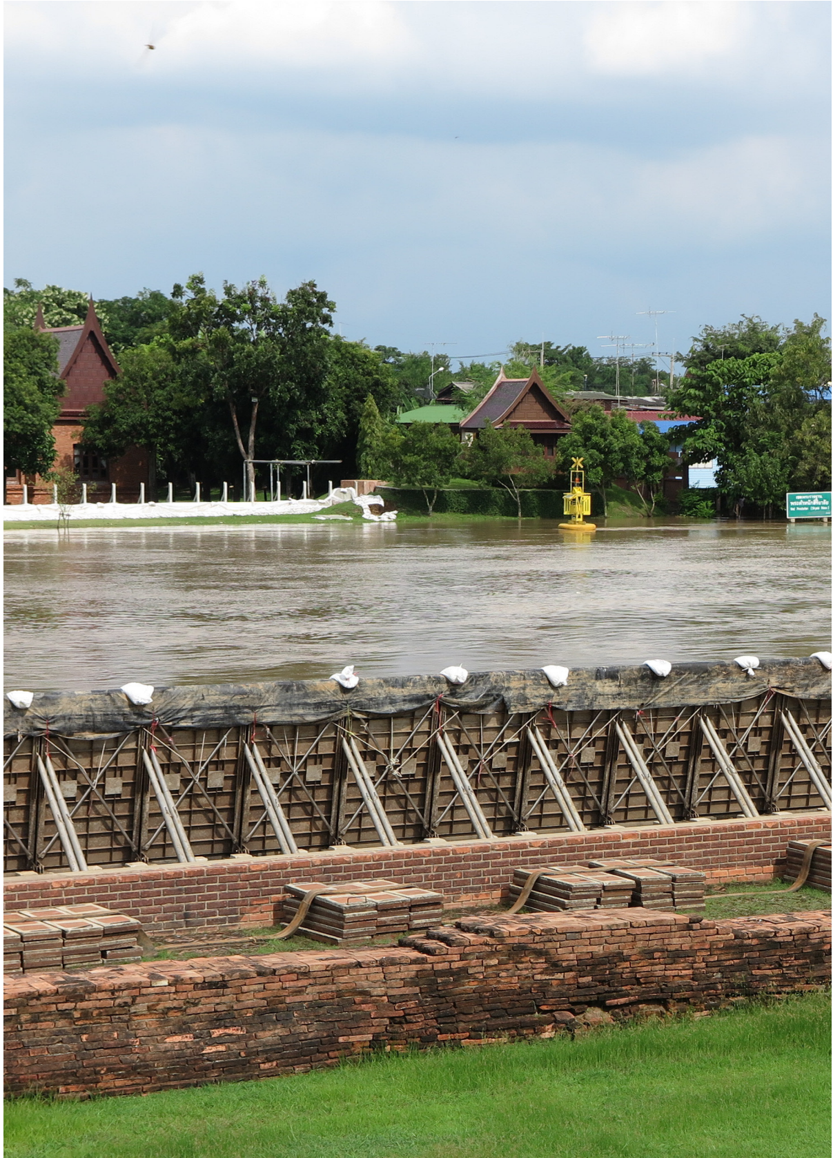
Dike, long wall or embankment built to prevent flooding at river near Wat Chaiwatthanaram, Ayutthaya historical park, Thailand Copyright: pawinpummarin. Retrieved from shutterstock.com
