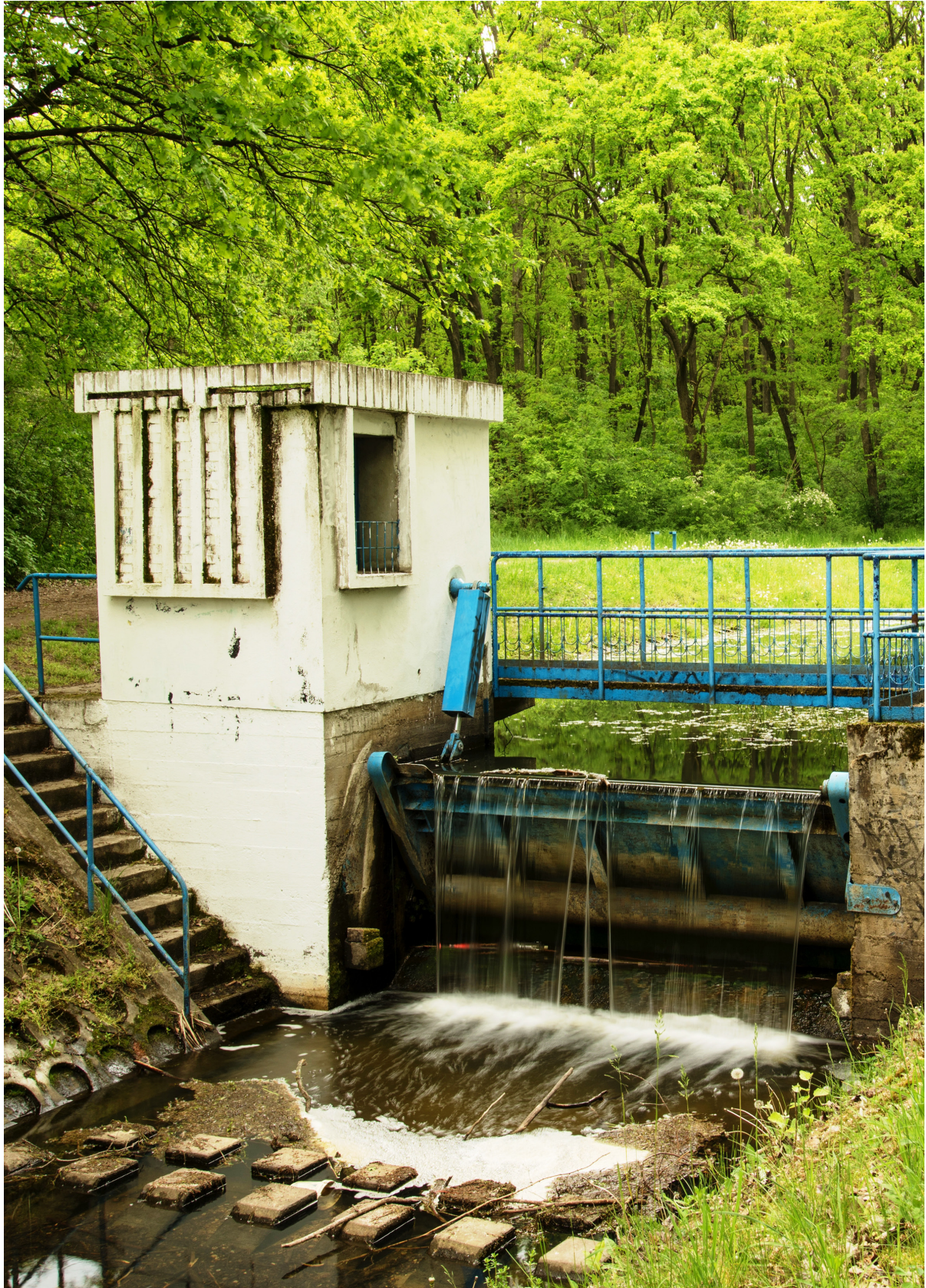
Flood gates of a small dam Copyright: Stieber. Retrieved from shutterstock.com
