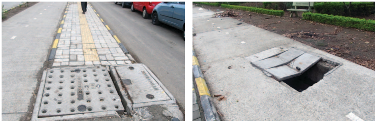
Figure 3.26 Inspection chambers on NMT lanes
