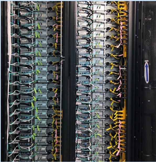
Figure 5. Tencent Liquid-Cooling Data Centre (source: Tencent)
